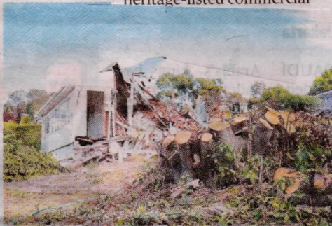
DESTROYED: Mt Stuart heritage home and tree
